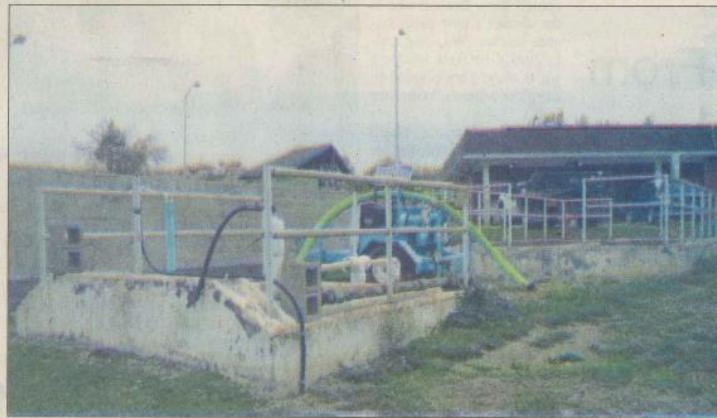
Sherman's aging sewer plant will soon have a new Direct Inline Pumping system installed.
